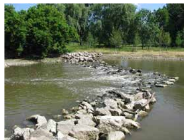
The relocated stream and constructed rock vanes channel water towards the center of the stream, reducing erosion.
