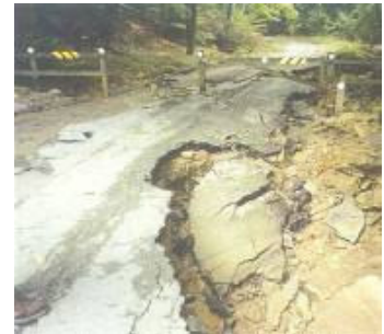
Stream overflows resulting in closing of the park road
